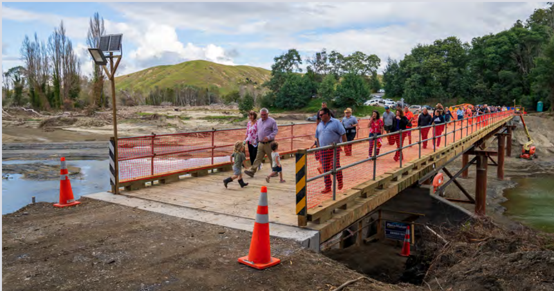
Opening of the temporary bridge that connects Dartmoor community with Napier. Photo credit: Mark Henderson/Hastings District Council.
