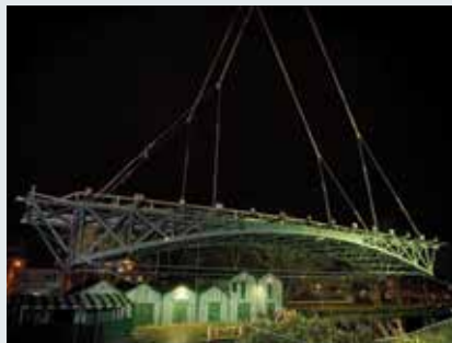
The Antigua Street footbridge is lifted out of its position and taken away for earthquake repairs.
