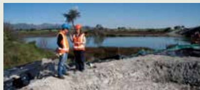
Omar Seychell from Fulton Hogan and Fiona Nicol from Environment Canterbury discussing erosion and sediment control for the cement grouting at the Bridge Street site.
