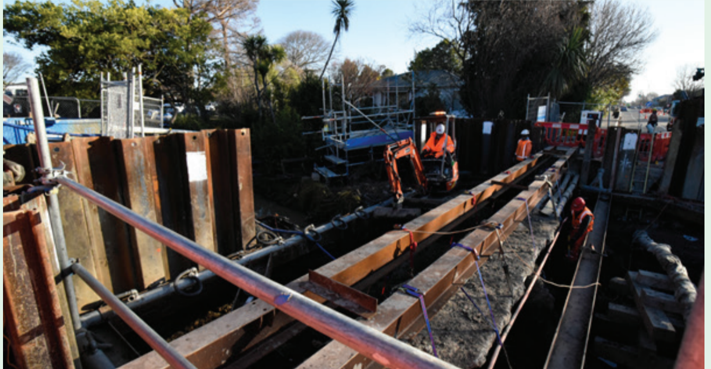
Work is underway to upgrade the Shirley Road stormwater culvert – part of the Dudley Creek upstream work to ensure floodwaters can be quickly taken away from the Flockton area.
