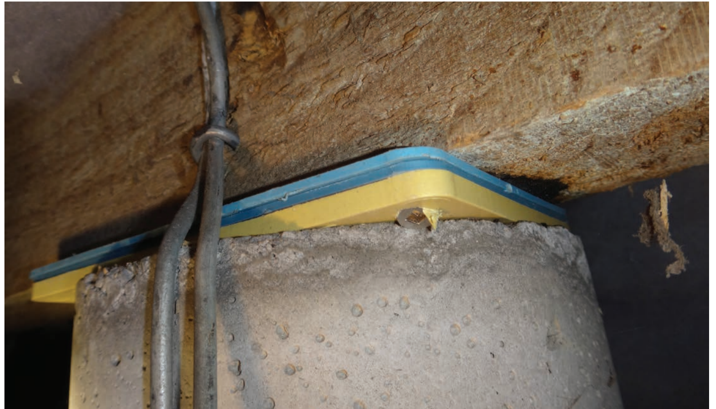
Example of compliant 'jack and pack' with packers fixed to bearers and piles fixed to timber bearers.
