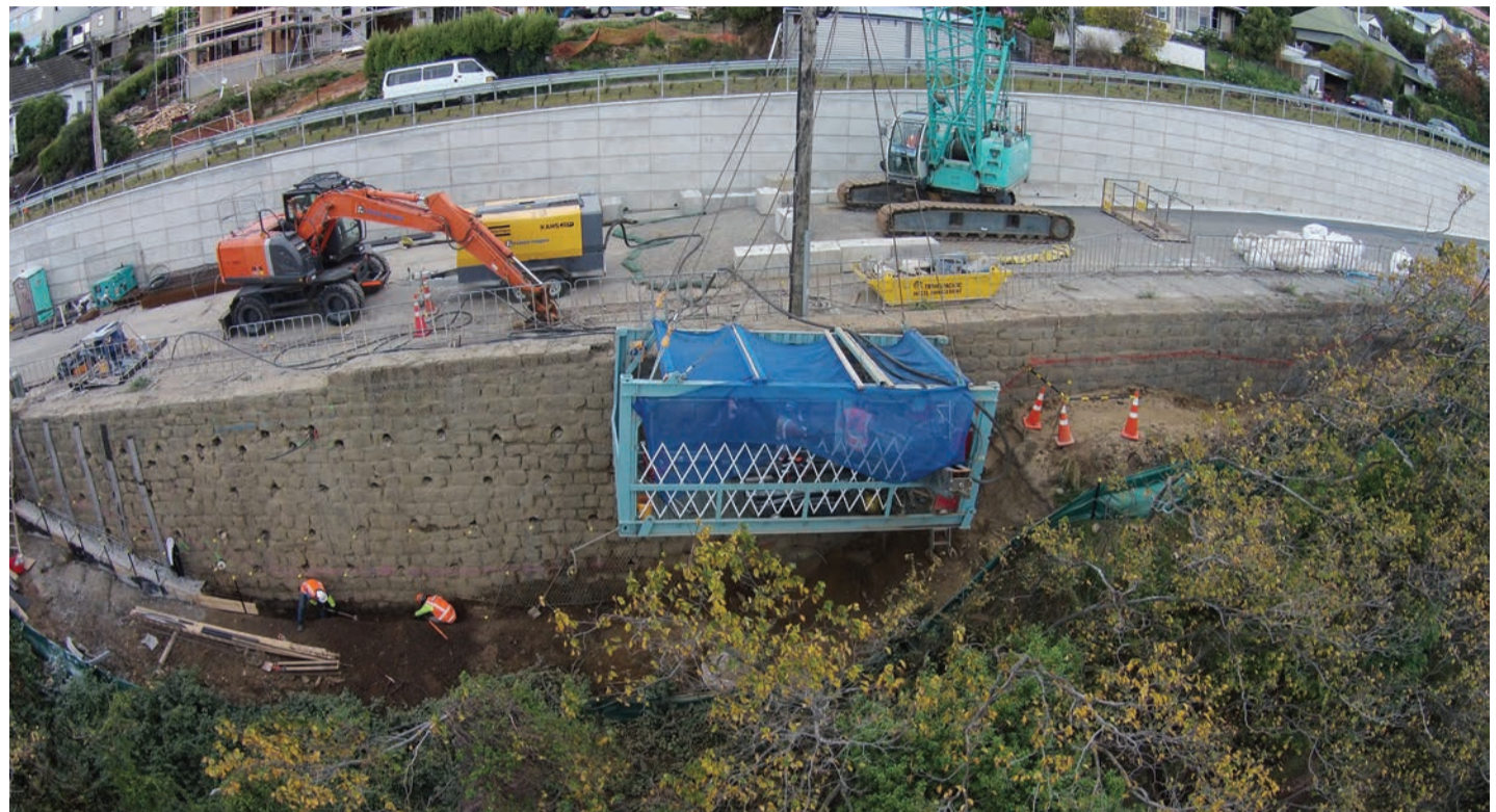
A day in the life of the SCIRT Fulton Hogan team repairing Lyttelton's Sumner Road retaining wall means working from a purpose-built platform suspended over the side by a crane. This essential earthquake repair project includes drilling over 170 holes in the wall to install 8-metre-long engineered reinforcing rods.
