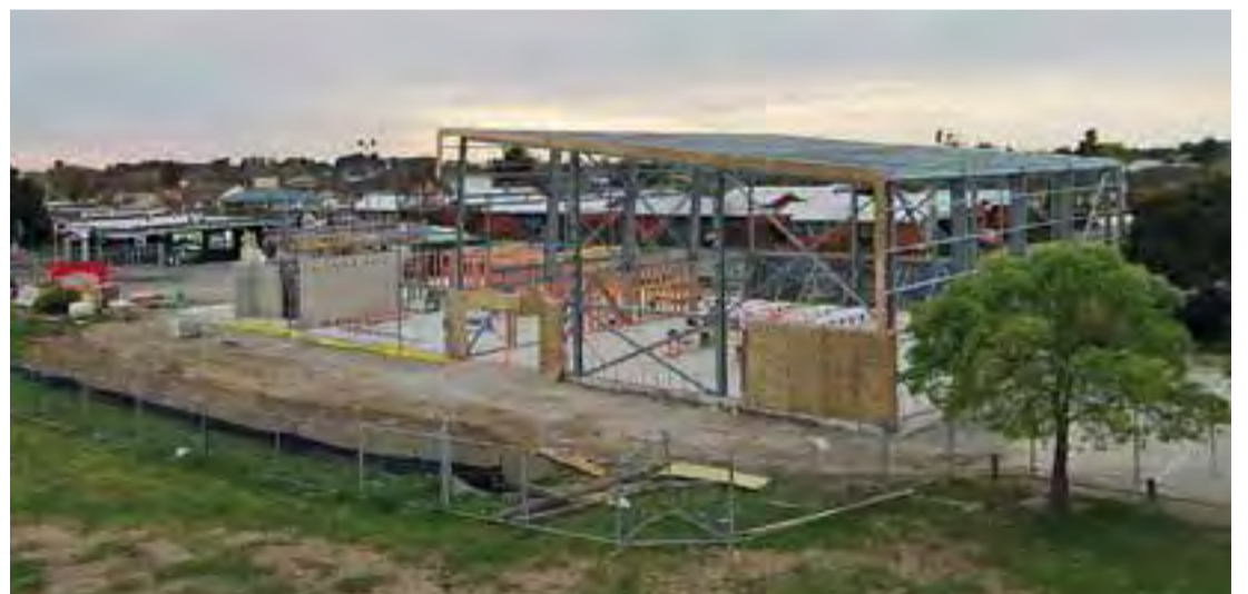
The structural steel work for the new Aranui Community Centre is finished.
