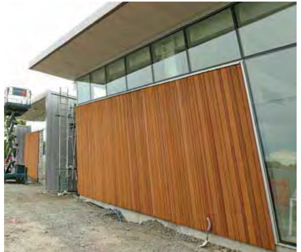
Sloping walls are a feature at the centre, as work continues ahead of the opening on 28 November.
