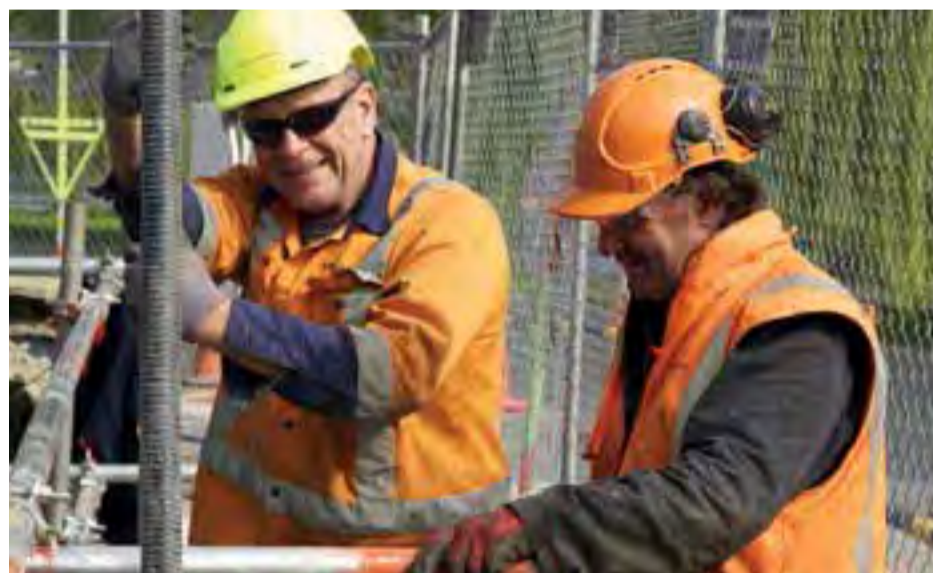
Jon Kissel and Warren Hoffman from SCIRT's City Care team working on one of Christchurch's wastewater lift stations as part of the overall network repair work.
