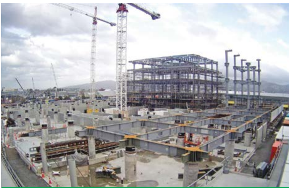
View of the site on 29 April 2015, showing the columns and base isolators.
