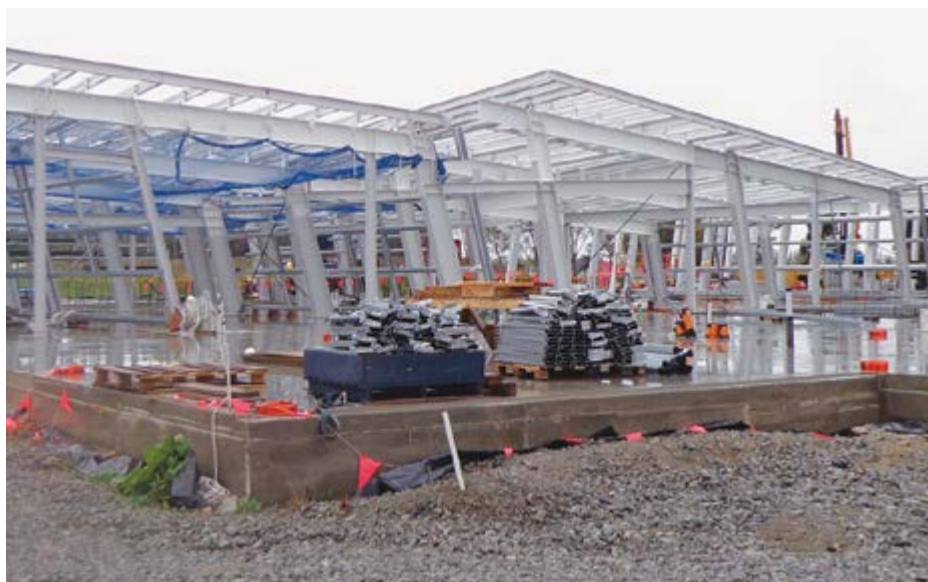
Construction underway on Te Hāpua: Halswell Centre. The steel frame is up and the roof has just been put in place.
