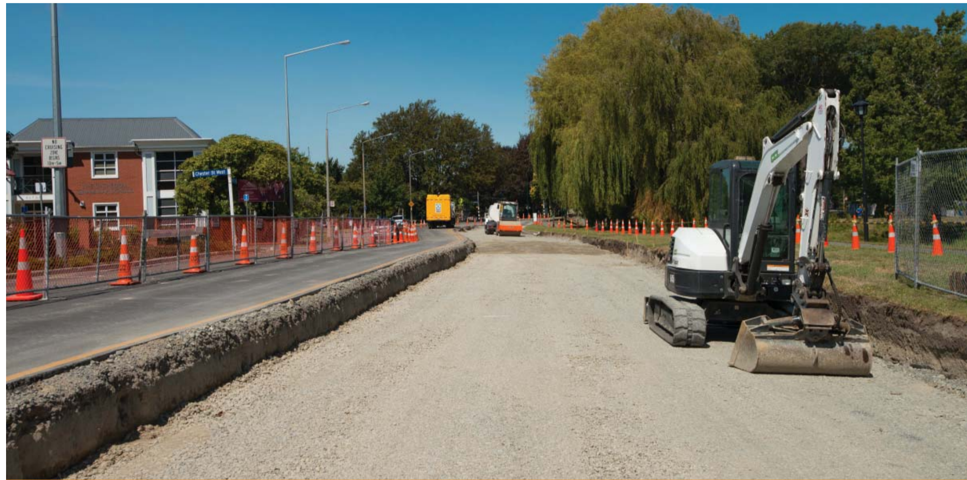
A substantial portion of Park Terrace was partially rebuilt as part of SCIRT's roading programme.
