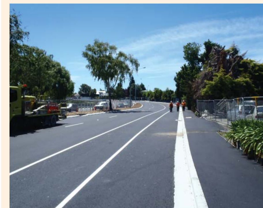
A large section of Fitzgerald Avenue was fully rebuilt after severe damage from the earthquakes.
