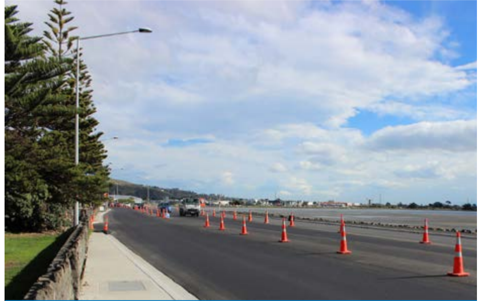
SCIRT's Fulton Hogan team were busy finishing work on Main Road, between Scott Park and McCormacks Bay Road, last month.
