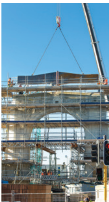
A strengthening top beam is lowered into the Triumphal Arch of the Bridge of Remembrance.
