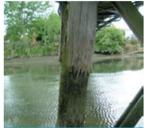
Catherine Street footbridge's piles showing signs of significant deterioration.
