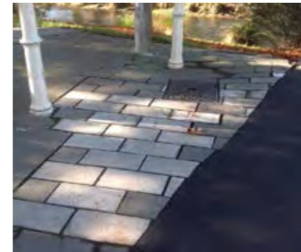
1 Uneven surfaces, broken pavers.
