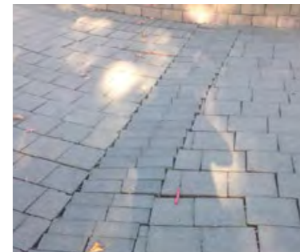
20 Lateral spread damage to paving.
