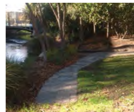
29 Earthquake slumping damage and unusable ground condition.
