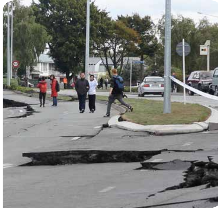
Fitzgerald Avenue road damage
