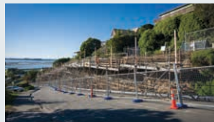
Soleares Avenue re-opened to traffic in September after a 10-month rock stabilisation project.
