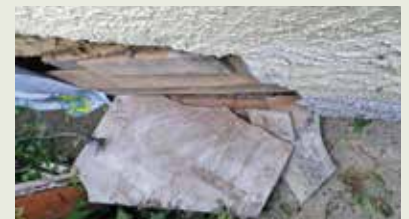
An example of asbestos board being found under house cladding.
