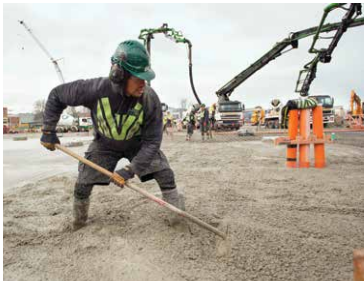
Hard at work: The foundation for the Bus Interchange takes shape. The Interchange is being constructed in a joint venture between Australian company Thiess and Christchurch's Southbase Construction.
