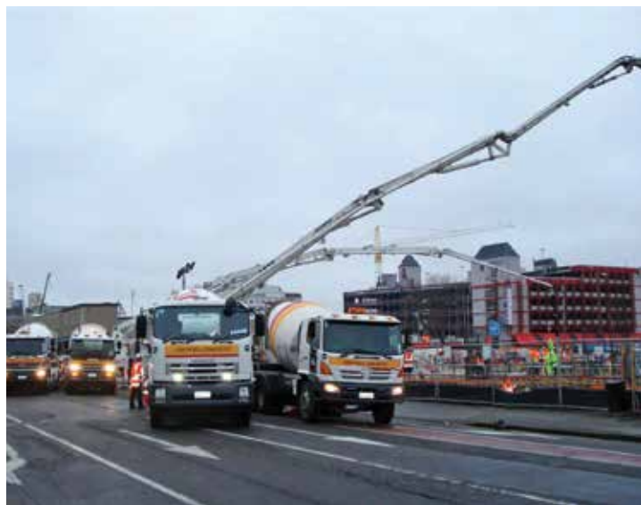
Trucks last month bringing concrete for the first pour for the main foundation slab of the Justice and Emergency Services Precinct. The operational car park will have its own foundation slab when construction starts at a later date.
