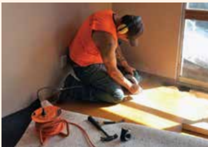
Pipi Schooner from City Care busy making repairs to a Housing New Zealand property in Buchanans Road.
