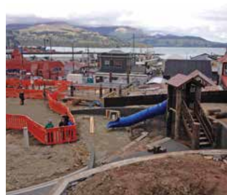
Work in progress: Albion Square on its way to becoming a focal point for Lyttelton locals.
