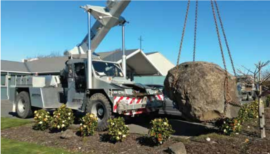
The Smith Cranes team delivers an 8.5 tonne Port Hills rock to its new Christchurch Chinese Church home.
