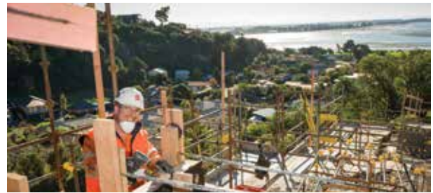
A worksite with a view - Lee Purves of SCIRT's Fletcher team working at the Soleares Avenue site.
