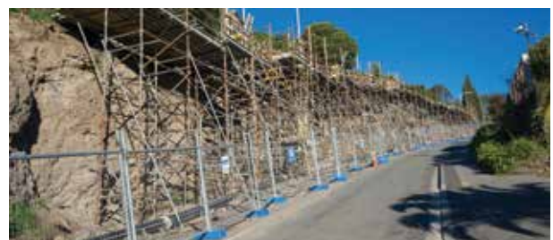
Major construction work was carried out on Soleares Avenue following the earthquakes to stabilise the rock face.
