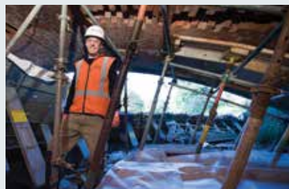
Tom Harding-Ilott, site engineer, with SCIRT's Downer Delivery Team working underneath the Armagh Street bridge.
