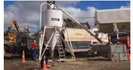
Not much to look at but the rectangular-shaped machine mixes tonnes of soil with cement for ground improvement at the Justice and Emergency Services Precinct site.
