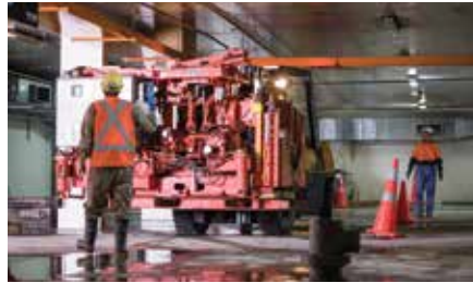
Complex foundation re-levelling work well underway. Image courtesy of Christchurch Art Gallery Te Puna o Waiwhetu.
