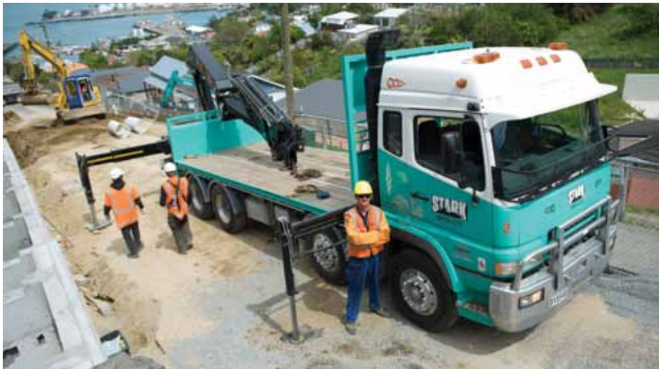
It's tough work rebuilding Lyttelton's retaining walls, but the setting for these SCIRT workers is hard to beat.
