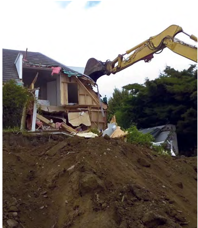
Complex and specialised land clearance work in the Port Hills will now be led by Land Information New Zealand.
