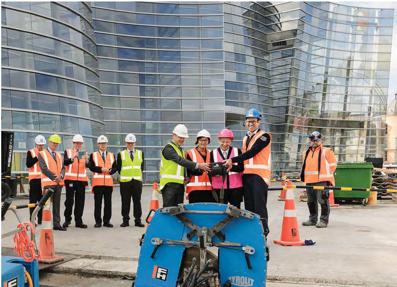
All together: Project Director Thomas Jones, Christchurch Art Gallery Director Jenny Harper, Mayor Lianne Dalziel and Fulton Hogan South Island Civil Operations Manager Ben Hardy push the button to complete the base isolation of the gallery building.
