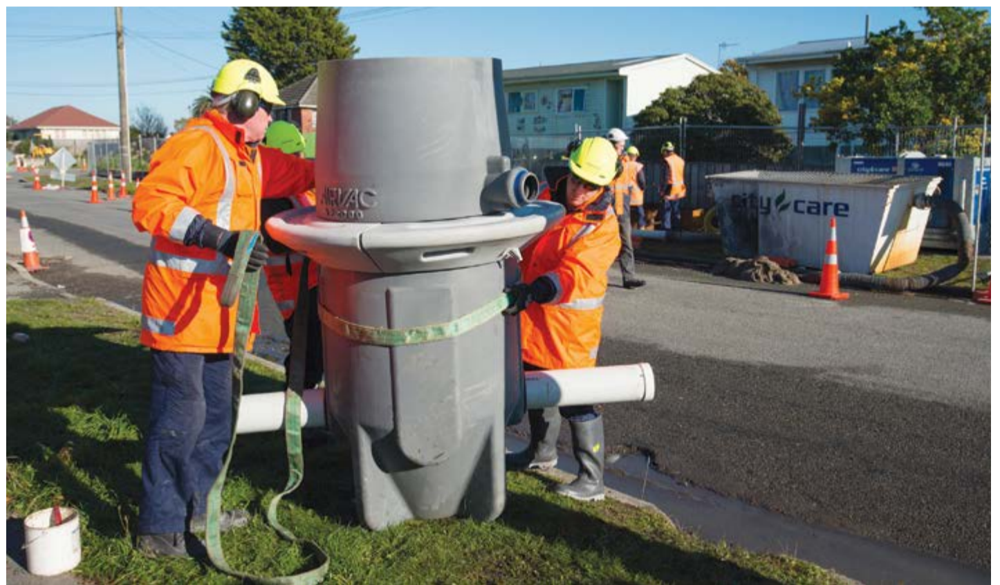
A SCIRT City Care crew busy installing vacuum wastewater chambers on an Aranui street.
