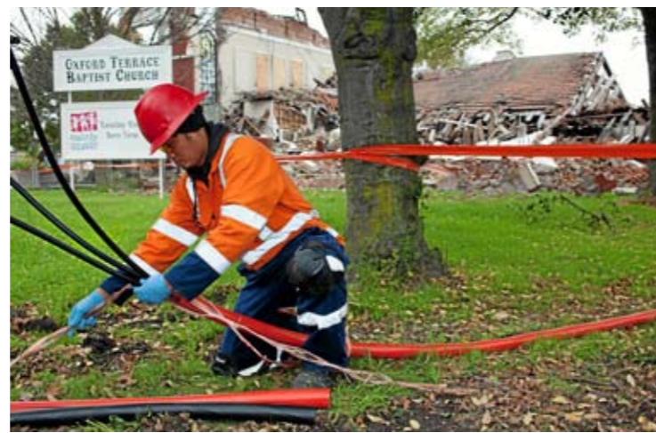
Ike Francisco from Counties Power in Pukekohe repairs damaged power cables in Madras Street.
