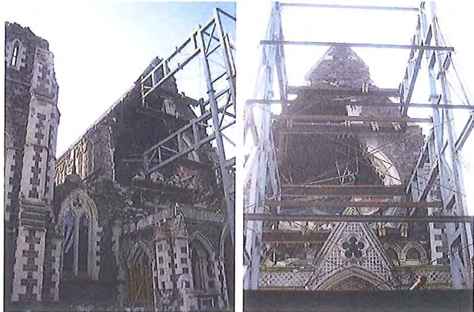
Figure 1 Damage Observed to the West Wall
