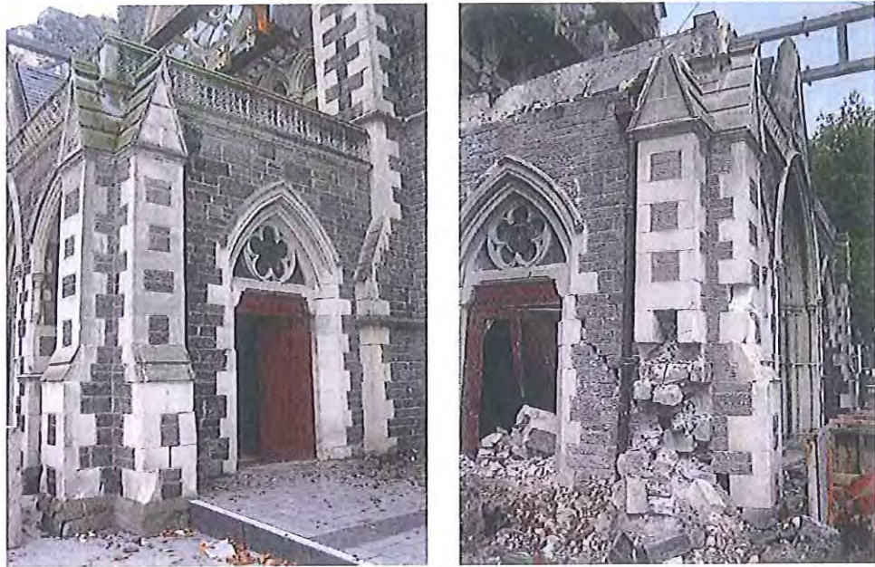
Figure 1 Damage Observed to the West Porch
