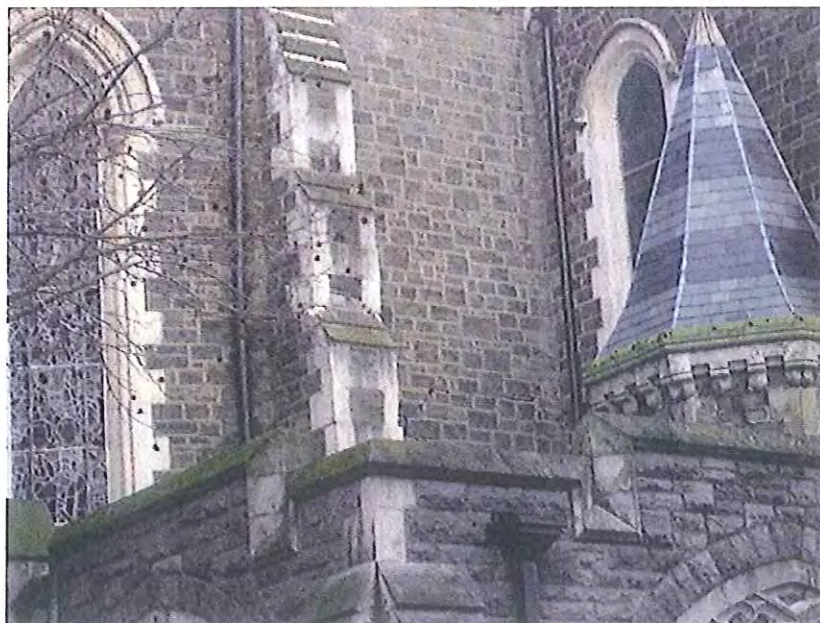
Figure 8 Damage Observed to the Apse North Wall
