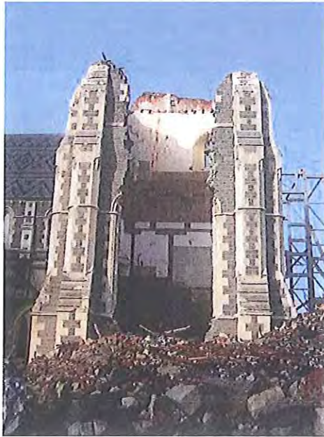
Figure 1 Damage observed to the Tower
