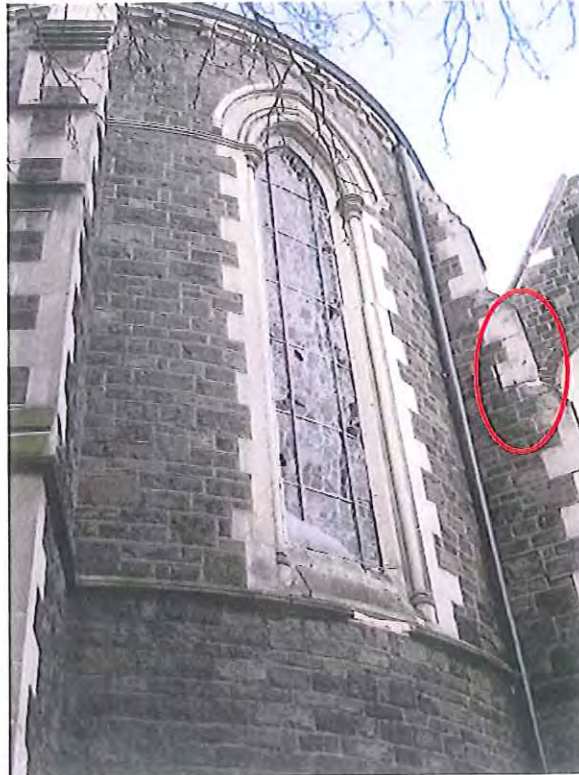
Figure 2 Re-check falling hazard above Clergy Vestry
