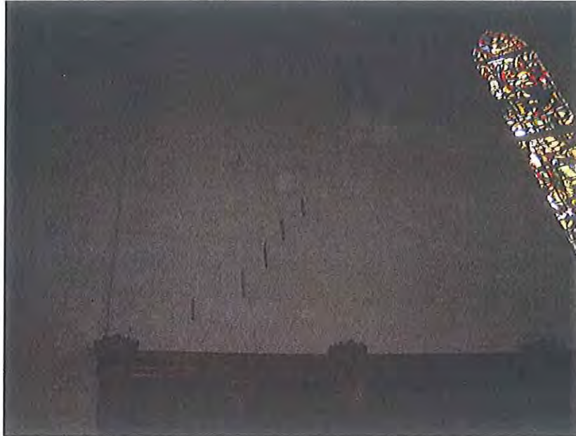
Figure 9 Interior View of Damage Observed to the Apse North Wall
