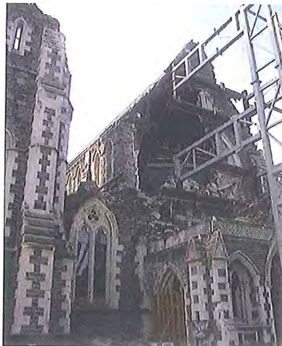
Figure 1 Christchurch Cathedral following June 13 th aftershock
