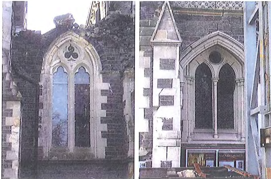
Figure 2 Damage Observed to the Hawdon (left) and West Porch Window (right)
