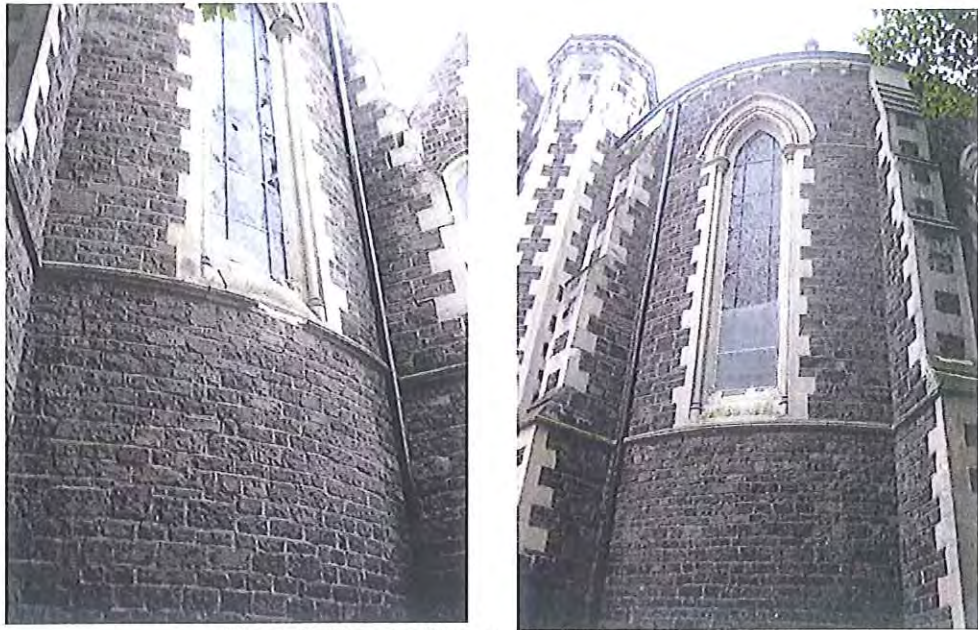
Figure 11 Damage Observed to the Apse
