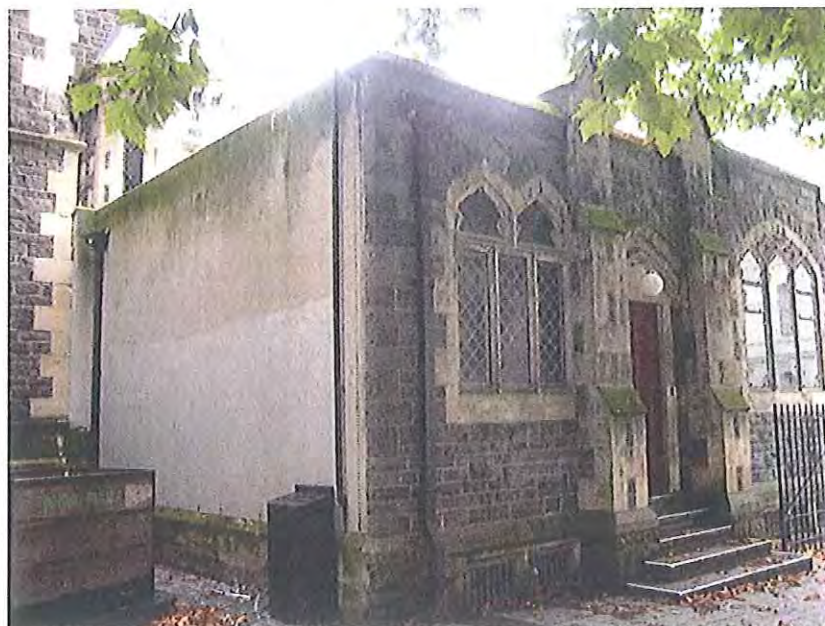
Figure 12 Damage Observed to the Clergy Vestry
