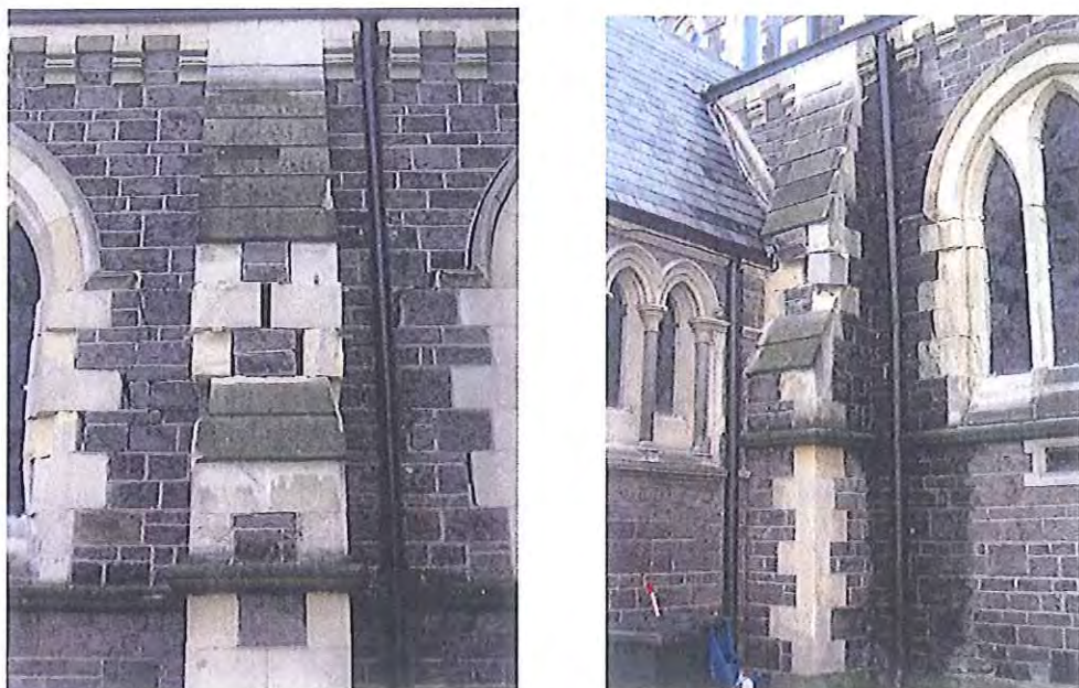
Figure 4 Damage Observed to the South Wall
