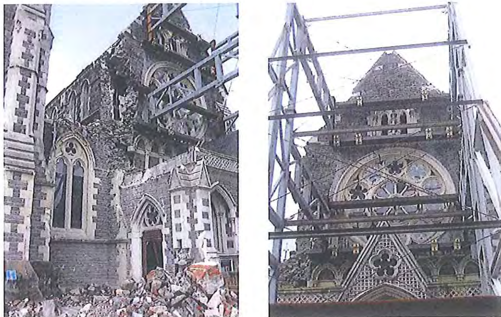
Figure 2 Damage Observed to the West Wall
