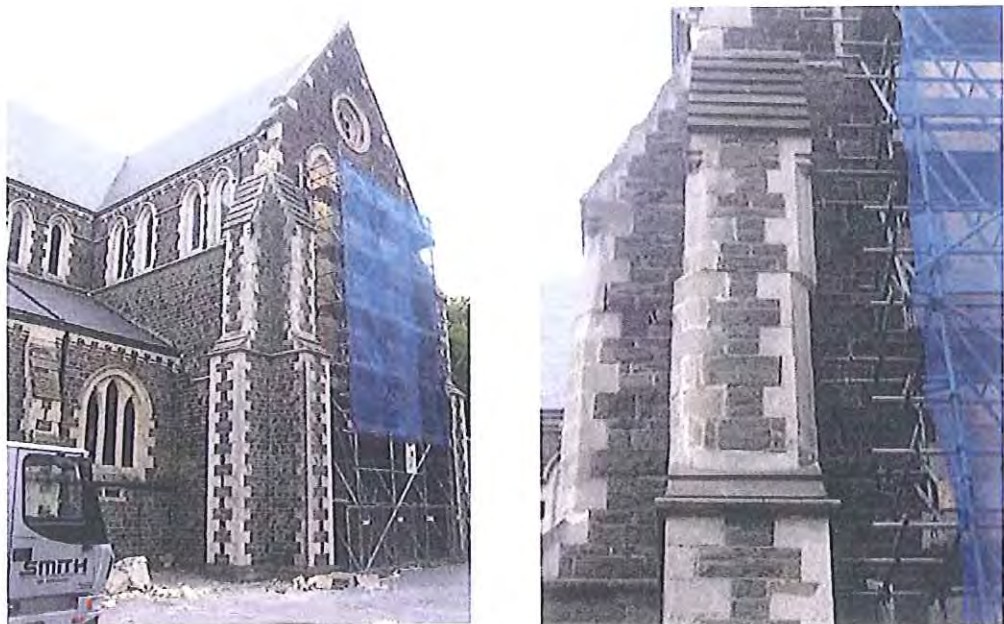
Figure 10 Damage Observed to the South Transept Wall
