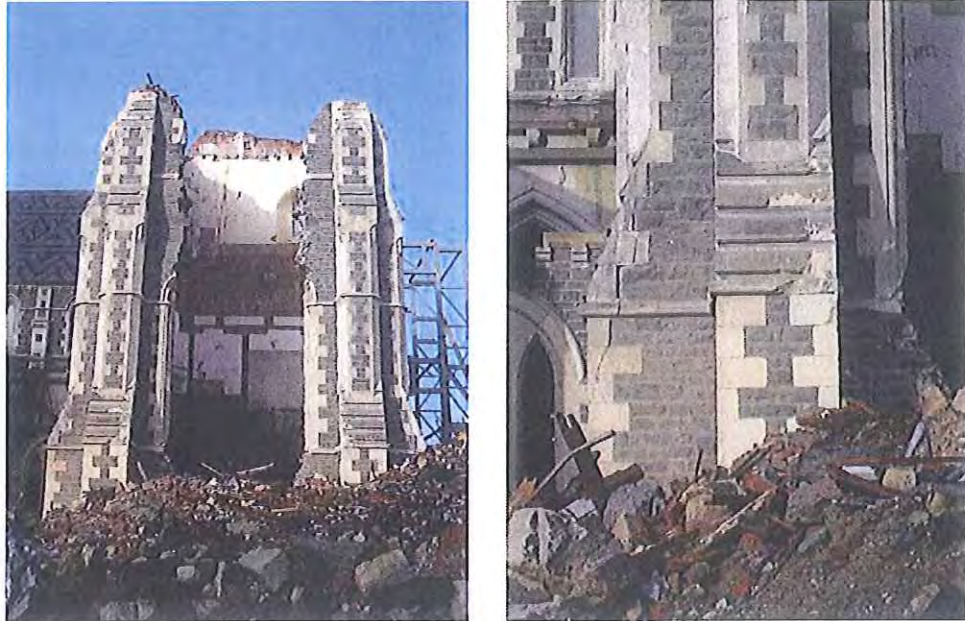
Figure 3 Damage Observed to the Cathedral Tower
