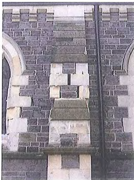
Figure 2 Typical damage pier observed to the south wall.
