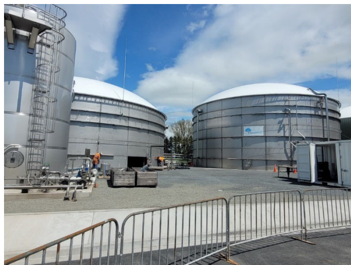
The digester tanks at Reporoa which hold up to 3,500,000 litres of organic waste. Methane rises to the top of the tanks and are captured using a hose system.
