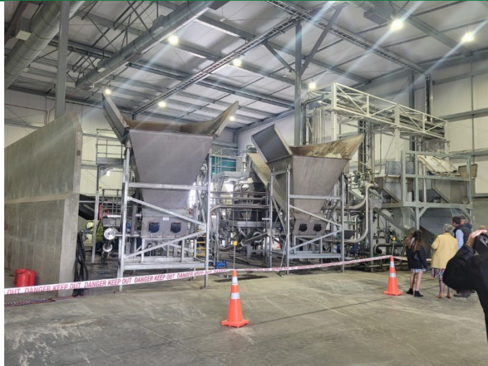
Sorting hoppers which receive and filter organic waste streams at Ecogas' Reporoa plant.
